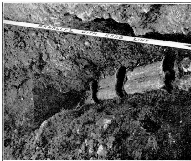
FIG. 2.—BOUGHTON HILL. STATE OF DUCTS ABOUT 20 YARDS FROM MANHOLE.
