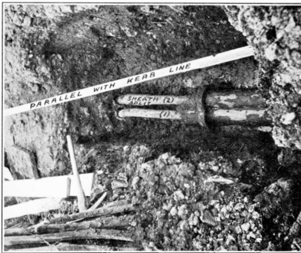
FIG. 3.—BOUGHTON HILL. DUCTS NEXT TO MANHOLE AT BOTTOM OF HILL.
