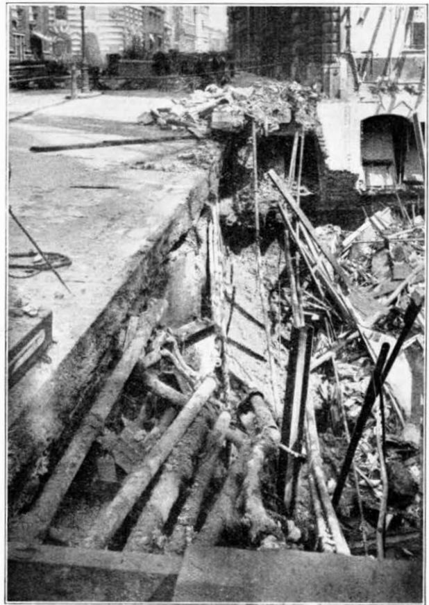
FIG. 1.—SITE IMMEDIATELY AFTER COLLAPSE OF BUILDING.
