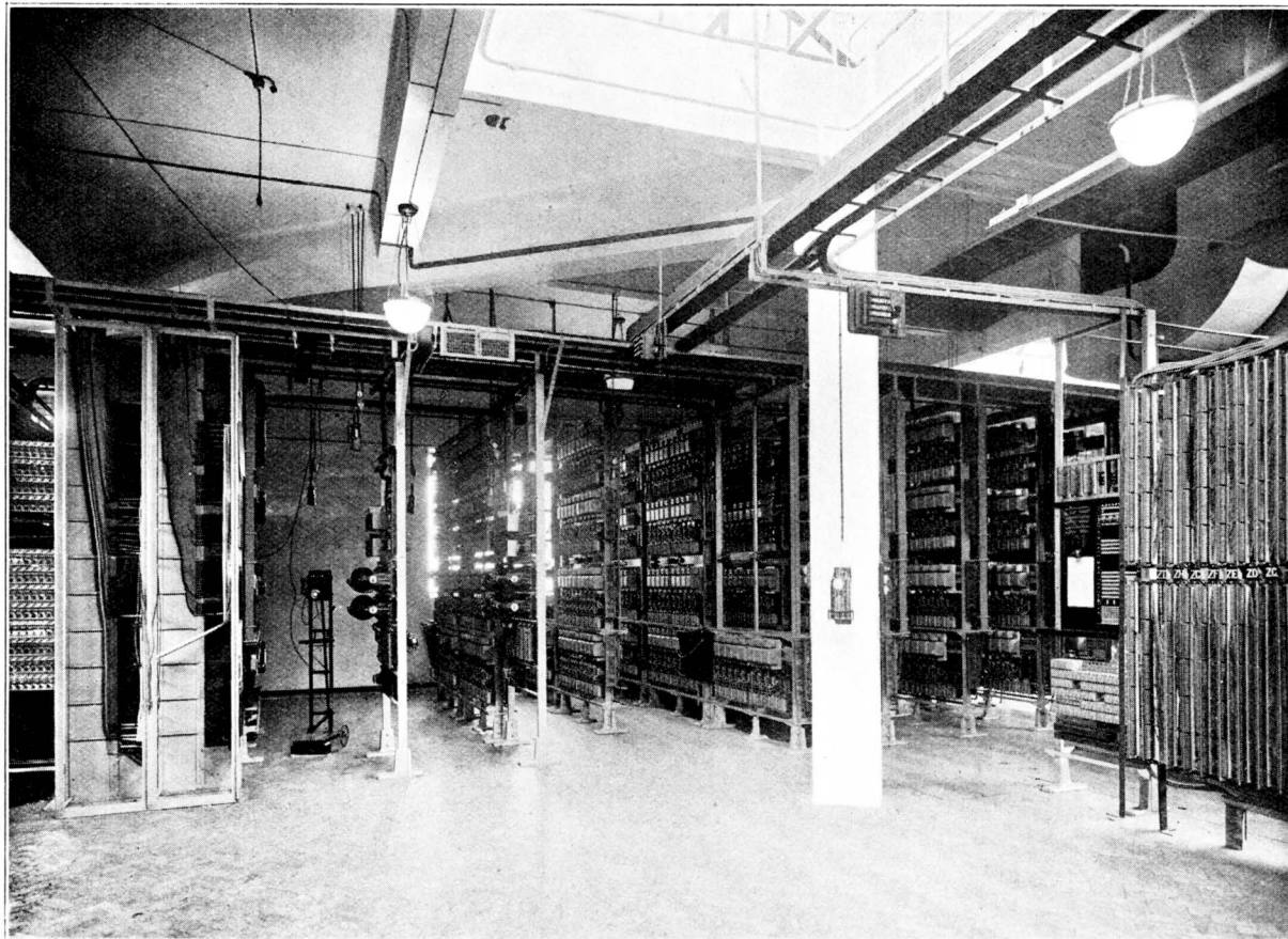
FIG. 5.—CENTRAL EXCHANGE, SHEFFIELD, FIRST SELECTOR RACKS.
