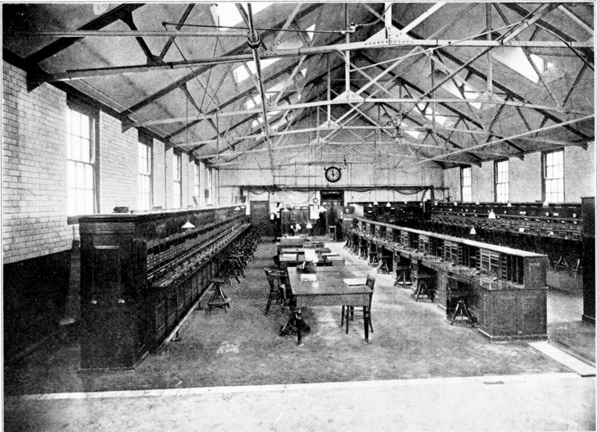
FIG. 1.—TRUNK EXCHANGE, SHEFFIELD. A AND J.E. POSITIONS ON LEFT. ENQUIRY IN CENTRE.
