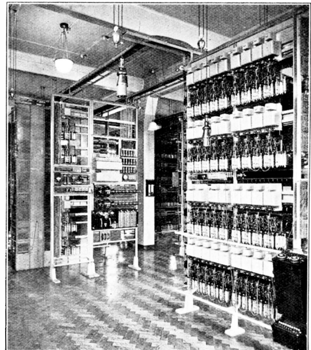
FIG. 4.—SHARROW EXCHANGE. FIRST SELECTOR RACK AND MOTOR-DRIVEN INTERRUPTERS.
