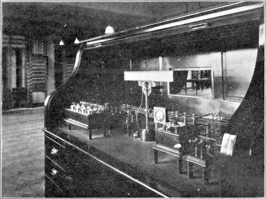
FIG. 26.—CABLE TEST DESK.
