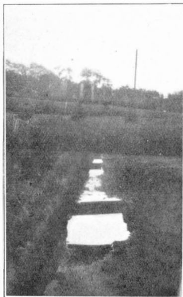
FIG. 7. CONDITIONS UNDER WHICH 75% OF WORK CARRIED OUT. RAIN AND DRAINAGE WATER ACCUMULATED IN TRENCH.
