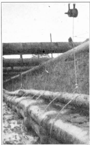
FIG. 6. DUCTS LOWERED INTO FINAL POSITION. C.I. PIPES ON RIGHT IN ORIGINAL POSITION.
