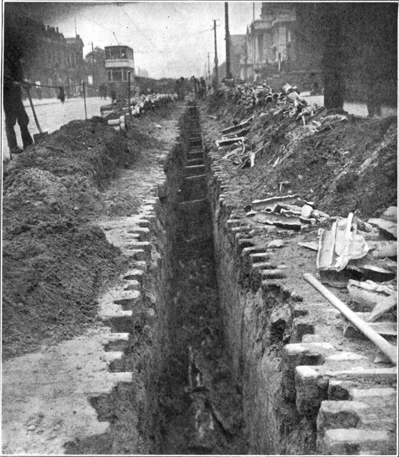
FIG. 2. CONDITION OF DUCT LINE AFTER EXPLOSION.
