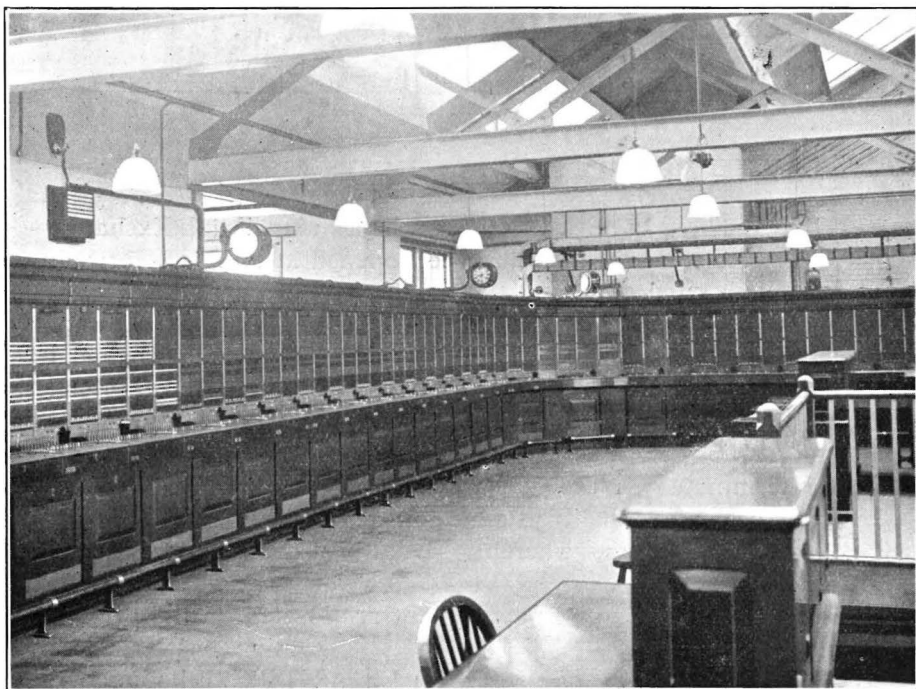
FIG. 1.—PART OF MAIN SWITCH ROOM. 25 SECTIONS ARE ON GALLERY ON RIGHT.
