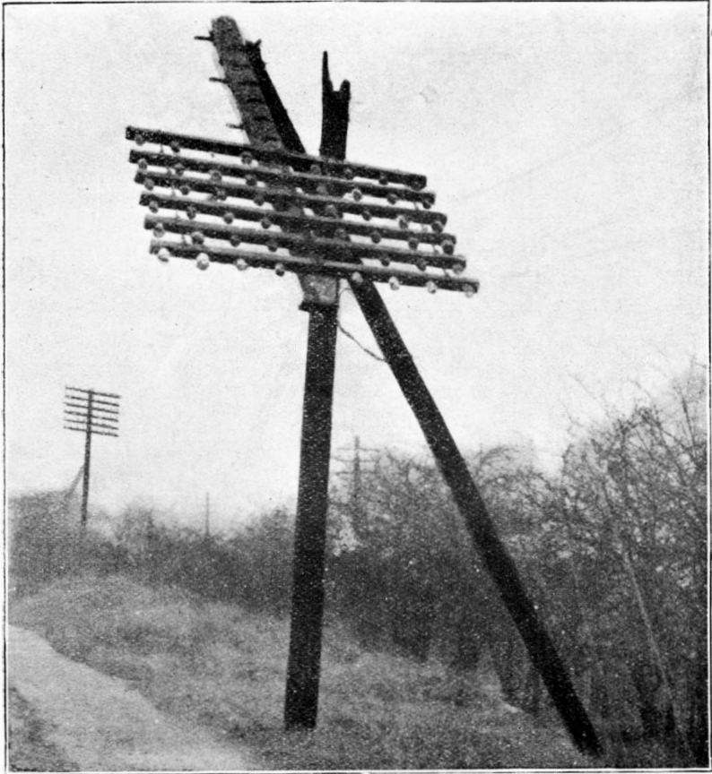
3.—LOCAL LINE, ALONG CANAL BANK BETWEEN BROOKLANDS AND TIMPERLEY. PRACTICALLY ALL DOWN FOR ABOUT A MILE.
