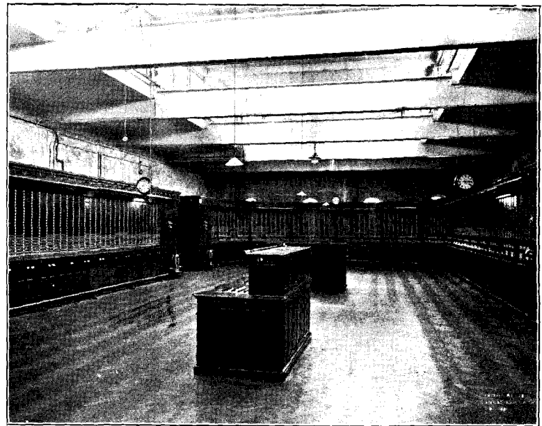
FIG. 11.—MIDLAND EXCHANGE SWITCHROOM: GENERAL VIEW.
