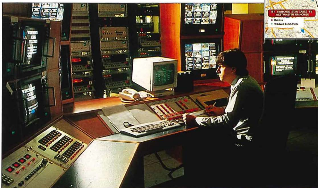
Left: Westminster Cable's control room.
