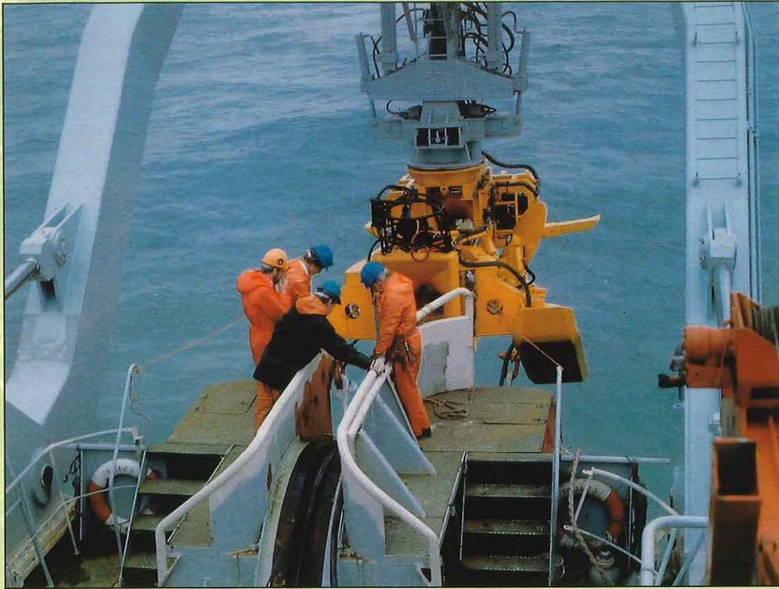
Left: British Telecom's Plough will be used to bury sections of the TAT 8 cable beneath the sea bed.
