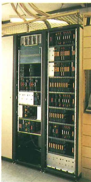
UXD5. British Telecom's new rural digital exchange.
