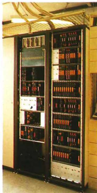
UXD5. British Telecom's new rural digital exchange.
