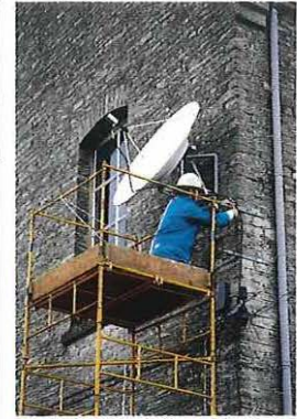
Small satellite dishes of the type attached to this building are likely to become a familiar sight on High Street betting shops.
