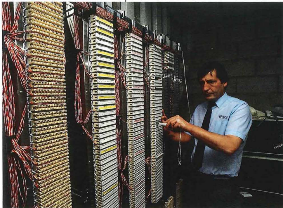
Senior technician Ricky Wilson working on a PBX built under Meadowbank Stadium to receive a 1,200 pairs cable from nearby Abbeyhill exchange.
