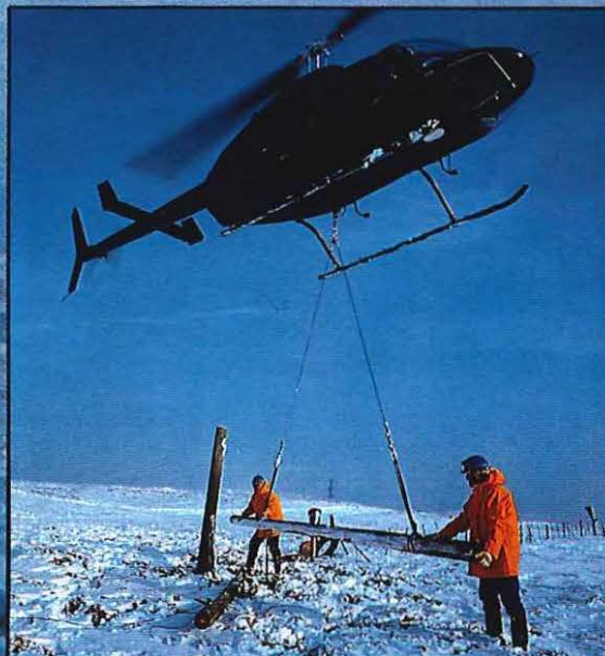
As usual, conditions in the Highlands of Scotland were particularly chaotic and this year British Telecom made use of a helicopter to fly in engineers, telephone poles and cable drains. These pictures capture some of the activity amid the desolation.
