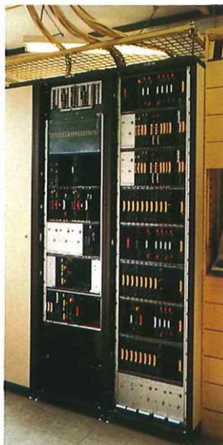
UXD5. British Telecom's new rural digital exchange.
