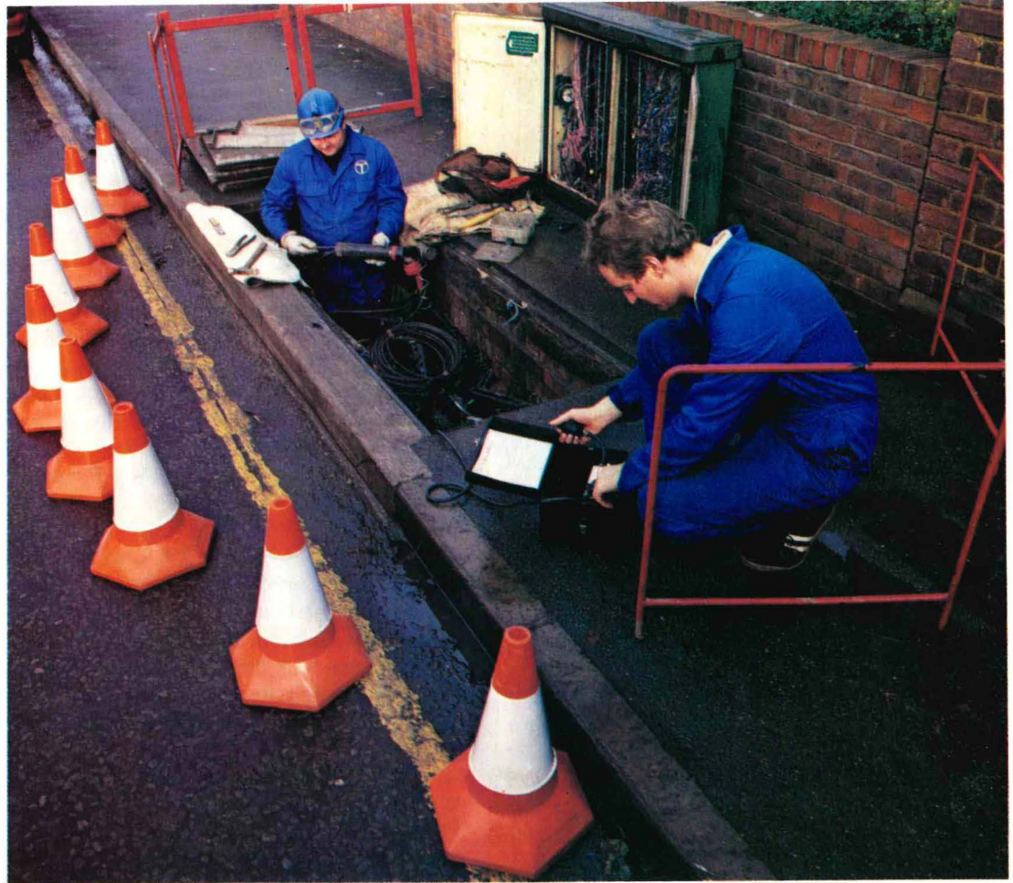
Engineers start work on a joint box to bring it up to modern standards. Dave Pepper (foreground) re-checks the readings of a gas analyser whilst Chris Slade replaces an obsolete joint.
