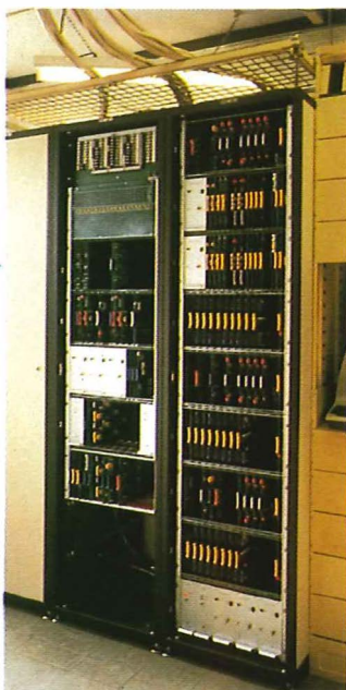
UXD5. British Telecom's new rural digital exchange.
