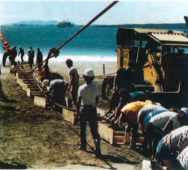
New Zealand engineers haul in a spur of the new Anzcan cable at Takapuna Beach, Auckland.
