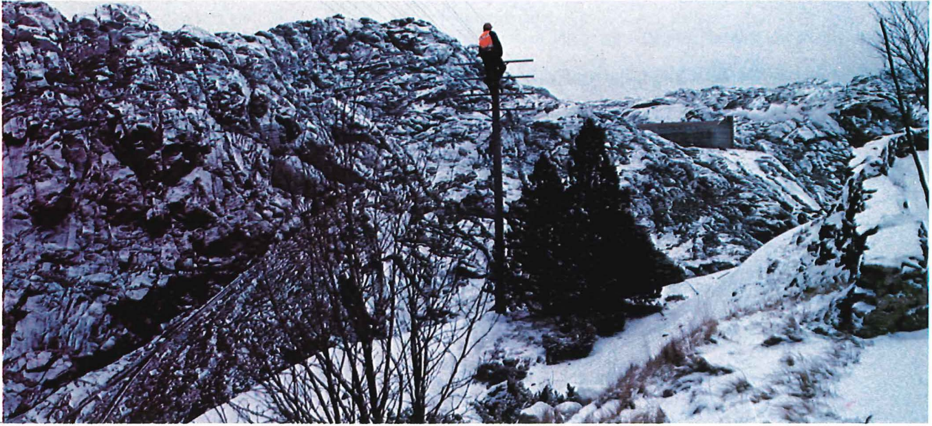
Maintaining overhead lines is a cold and lonely business in the Norwegian winter.
