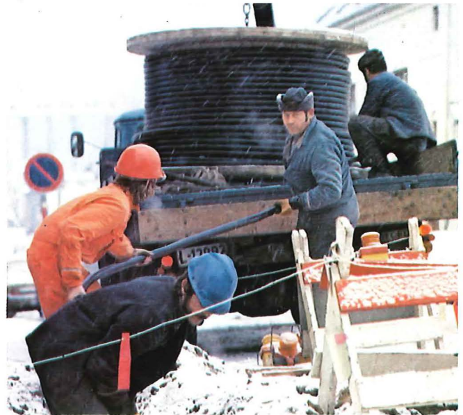
Norwegian technicians at work hauling in a new cable by the roadside.
