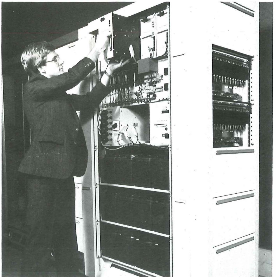
Design engineer Ray Kingdom replaces one of the five compact 28amp rectifiers in a power equipment rack (PER) being tested in London.
