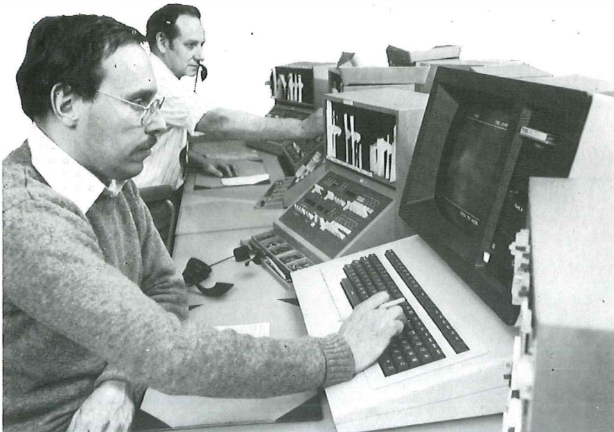
The remote line tester control and display provides invaluable information about conditions. Technical officer Mick Wheeler keys in a command for the computer to interrogate a line.
