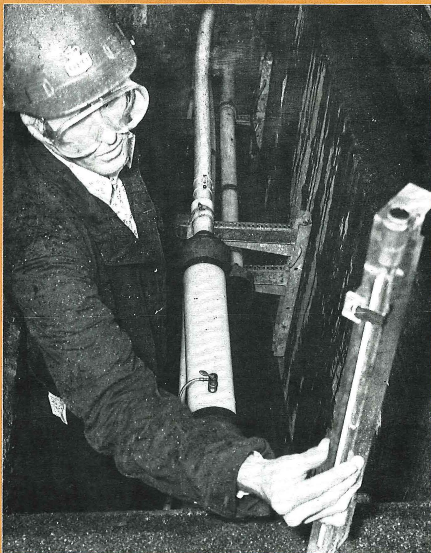
Polyethylene has been extensively used to insulate telephone cables throughout the British Telecom network for many years.
