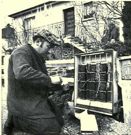
An engineer at a roadside cabinet connects a subscriber's line to the local telephone exchange.
