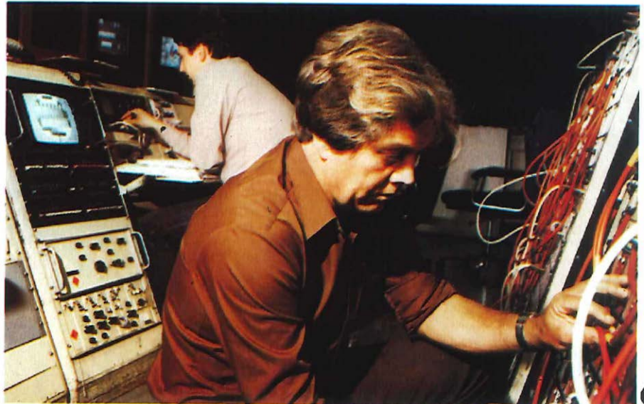
Bert Herring and Colin Harman patch a cord into the Crystal Palace circuit during a line test from the television switching centre at London's Telecom Tower in the heart of the West End.
