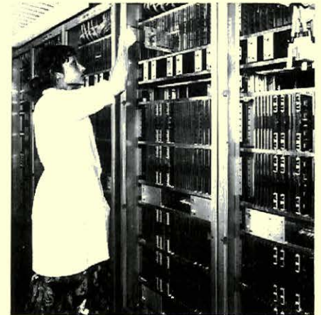
A technician inserts a printed circuit board at an electronic exchange.
