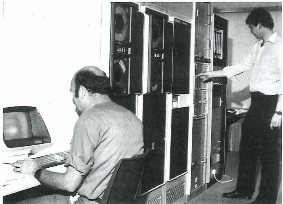
Clerk of works Dick Roynan (left) checks the status of the NCS simulator on the maintenance system which is part of the ACSE equipment being installed at Goonhilly.
