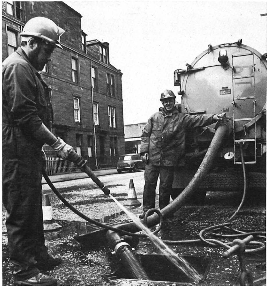
Flooded, sludge filled manholes are no longer a problem to British Telecom engineers following the arrival of new vehicles in Scotland which can suck out 2,000 gallons in about half-an-hour. The vehicles have twin 400 gallon tanks with one holding fresh water and the other used for collecting the slurry.
