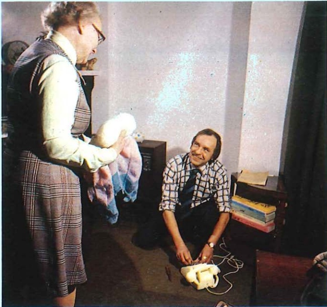
Every day, nearly 2000 telephones are installed by British Telecom to customers throughout the country. Maintenance is an equally vital factor and British Telecom's performance in this area is continuing to improve.
