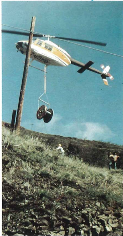
At a remote location near Hood River, Oregon, engineers from the Northwest Telephone Company of the Northwest 'string wire' with the help of a helicopter.
