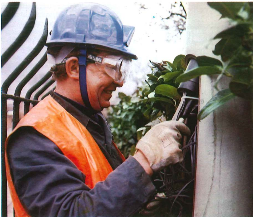
With a hollow pole, technician Len Pullen can work safely at ground level to replace the jointing sleeve after terminating a new dropwire. The potential danger of the railings to a man working at the top of a wooden pole was one of the reasons for installing a hollow pole at this site.
