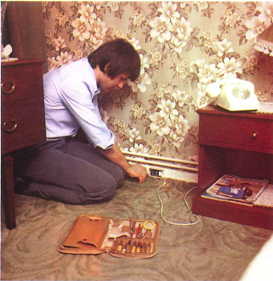
An engineer demonstrates the installation of the plug-and-socket system at a customer's home.
