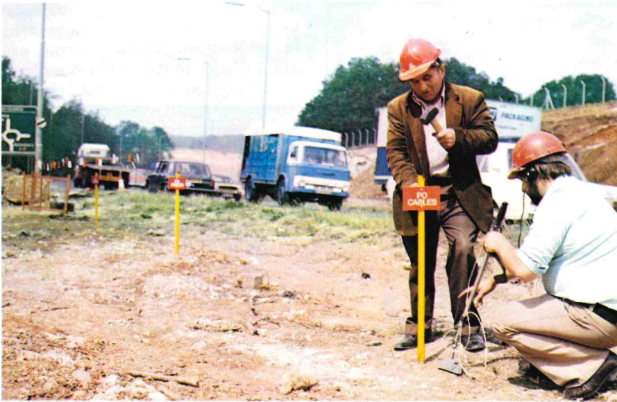
With the aid of special track locating equipment British Telecom staff are able to trace and mark the route of a telephone cable at a roadworks site.
