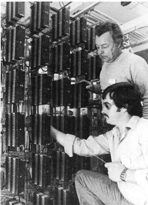
Like any other exchange, Airshow has its own main distribution frame. Technicians Ted Clifton (standing) and Trevor Dooner wire in another customer's line.
