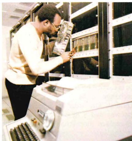
Technical officer O'Neil Bartley monitors a suspected faulty line terminator card at the St Botolph's stored program control gateway telex exchange. In the foreground, an unmanned teleprinter checks traffic patterns.
