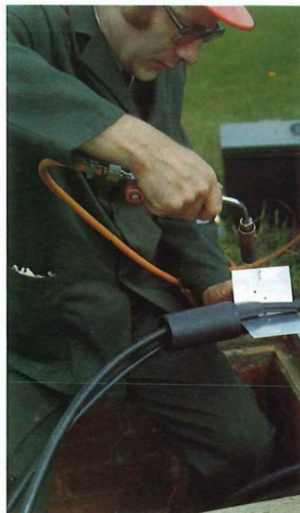
Above: Technician Dave Radford uses a specially designed tool to protect spare outlet ports as he applies heat to fix a multi-entry shrinkdown collar on to a cable.
