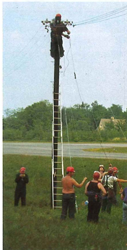
Above: A trainee at Moreton-in-Marsh begins tensioning the 200 pound copper wire used along the test route.
