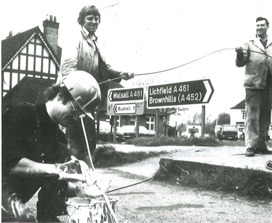
An optical fibre cable on the Walsall-Brownhills route is coated with lubricant to enable it to glide easily into the duct.
