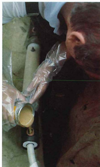
Below: Dave Cooke, a technician, pours resin into a mould before applying the shrinkdown sleeve between the joint sleeve and the block.
