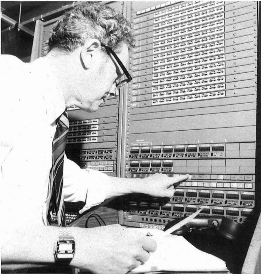
Above: Technical officer Ted Walton checks a call through the exchange in the basement of the Nat West building.
