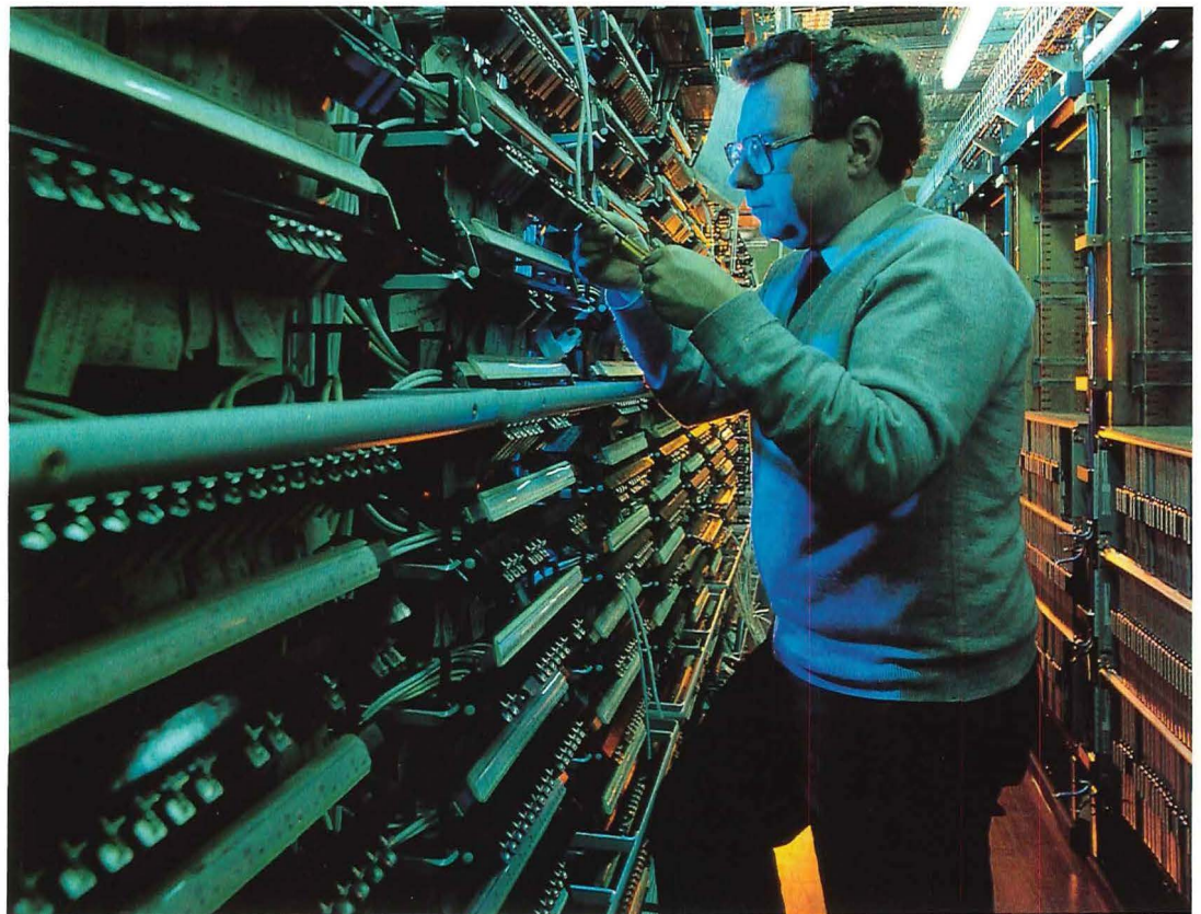
Right: the trunk network is constantly evolving – here an extension to the System X Digital Main Switch Unit (DMSU) is being installed at the Baynard House digital trunk exchange in London.
