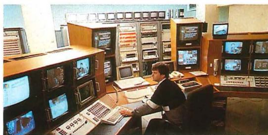
The control room at Westminster Cable TV.
