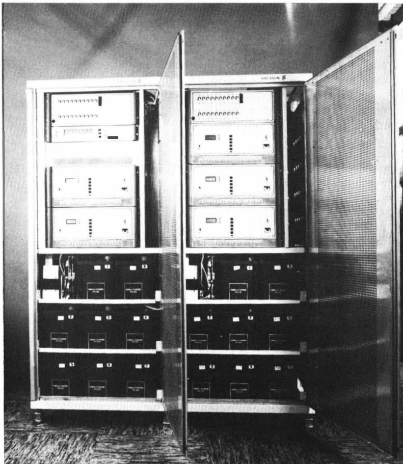
Figure 4—A pair of 5-shelf power cabinets
