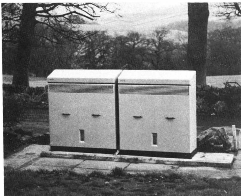
Figure 6 RSS 256 external cabinet installed at Wincle near Macclesfield
