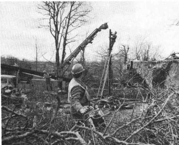
Repairing line damage caused by falling trees to restore telephone service to a remote farmhouse near Ruan Lanihorne in Cornwall
