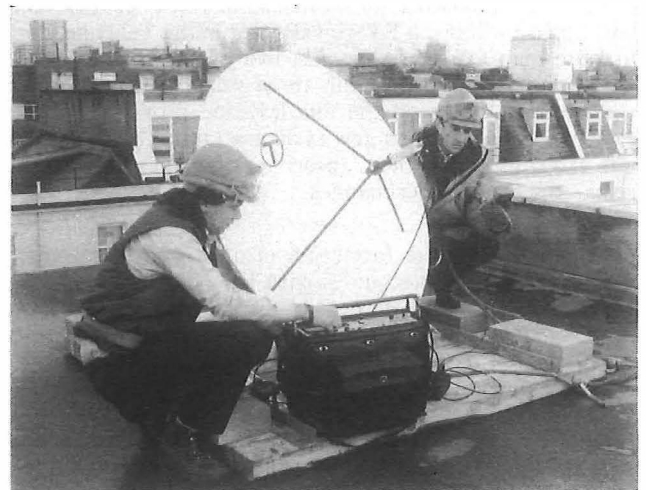
BT engineers installing and pre-testing satellite receiving dish equipment at a betting office site
