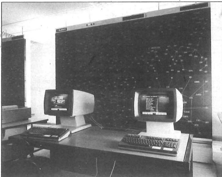
Figure 5 NMC display board
