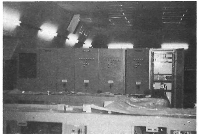
Fig. 10—Main control cubicles
