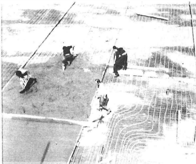
Fig. 1—Covering plastic pipes with concrete during the installation of the closed-loop heat rejection system at Sandridge Computer System
