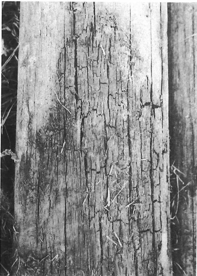
(b) Surface decay
