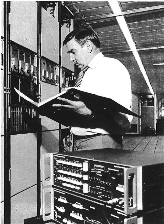
FIG. 2—Transmultiplexer installation at Keybridge House
