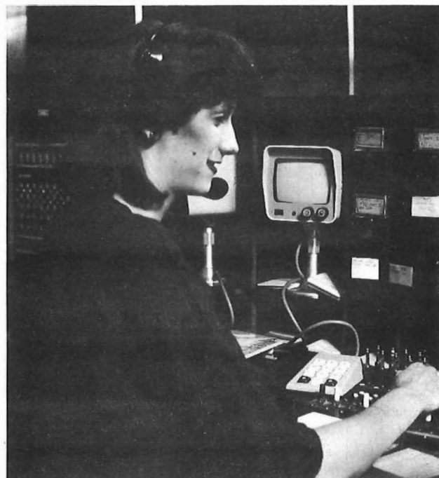
FIG. 1—Enquiry-operator position at Reading AMC equipped with a SEQUIN visual display unit and keypad
