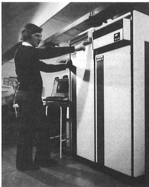
FIG. 1—TRIPOS installation at Leeds PCO
