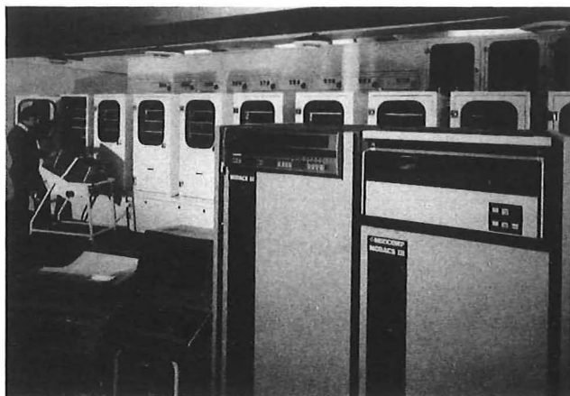
FIG. 2—Parcel-sorting-machine controllers adjacent to the TRIPOS installation at Leeds PCO.
