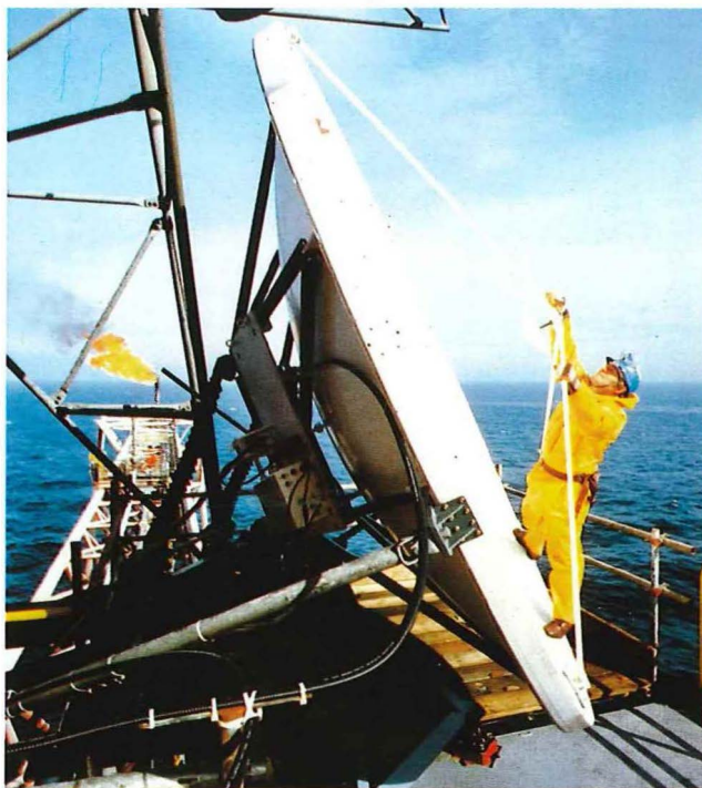
Installation of a small-dish antenna on the AMOCO Montrose Alpha oil production platform in the North Sea
