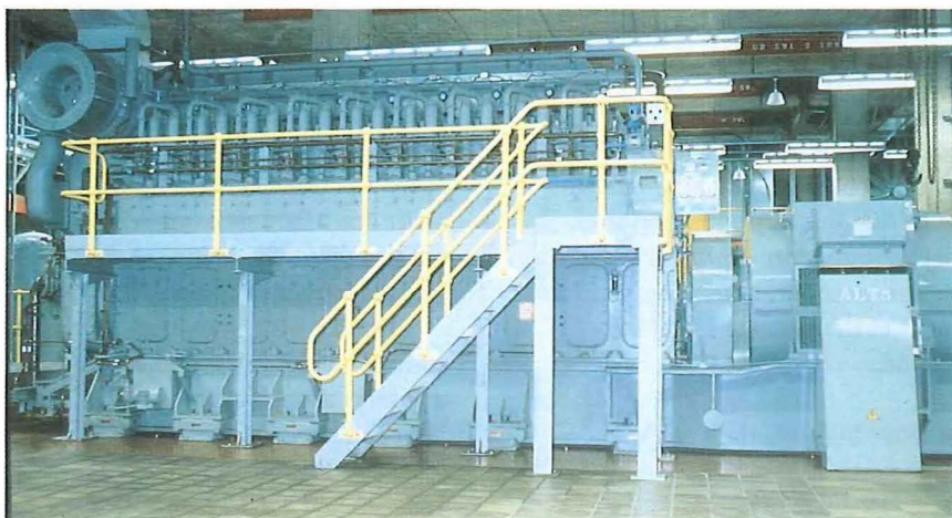
Figure 4—2.8 MW 11 kV generating plant
