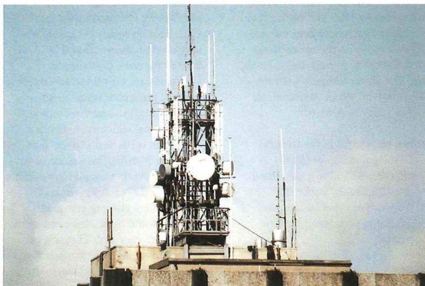
Figure 1—Mercury Communications Limited radio node structure on the Leeds skyline
