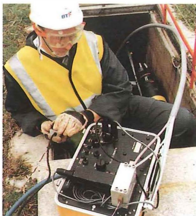
BT technician at the kerbside uses blown-fibre equipment to install optical fibre into the telecommunications network
