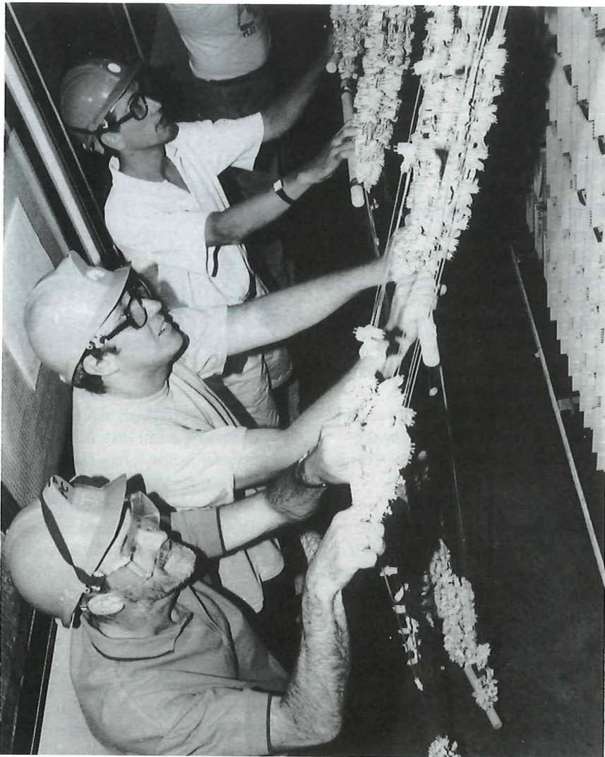
Figure 5—Exchange transfer—removing INTEST wedges on the MDF
