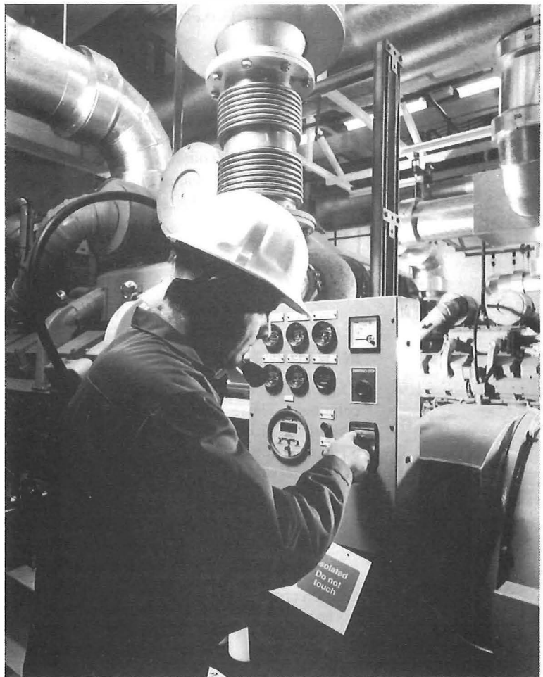
Figure 2 Permits to work and interlocks are an everyday part of power work
