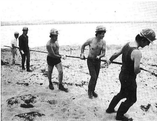
FIG. 13—Landing a subaqueous section of optical-fibre cable (Photograph courtesy of North-western Evening Mail)
