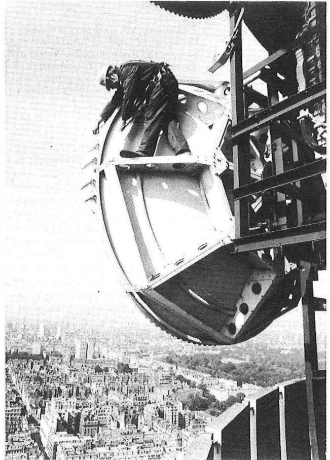
FIG. 2—Adjustments being made to one of the new dish aerals mounted on the London Telecom Tower
