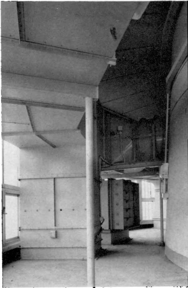
19 Plant room, level B3, showing one of the main extract fans and ductwork
